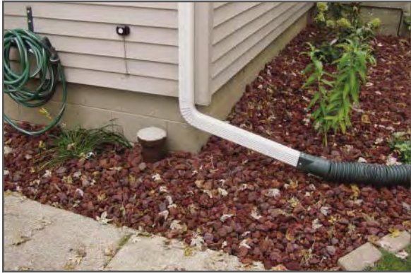
Redirected Downspout and Plugged Riser Pipe
