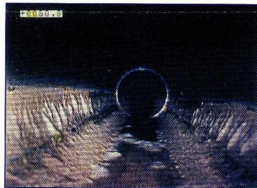
Although grease is a typical component of sewage, it can build up and cause blockages. Video inspection provides pipeline maintenance crews with a view of the inside of pipelines and the ability to detect problems such as the grease that is collecting on the sides of this pipe.
