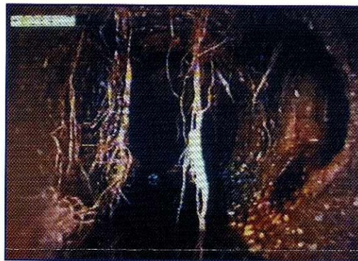
Roots, such as these found during a pipeline video inspection, can grow into pipes through joints and manholes and cause damage to the pipe. An aggressive program is in place to find and remove roots.
